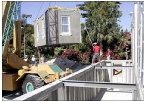
Picture: Glenn Tucker Built for speed: Construction workers get to grips with a section of the modular home that was built in just one day.
